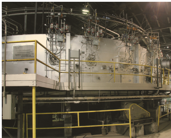
Fig. 10. Outside view of the rotary hearth furnace at ArcelorMittal Shelby after the conversion into all flameless oxyfuel operation. Please note that all bulky equipment and piping relating to the previously used air-fuel system have been removed as it no longer is of any use.
